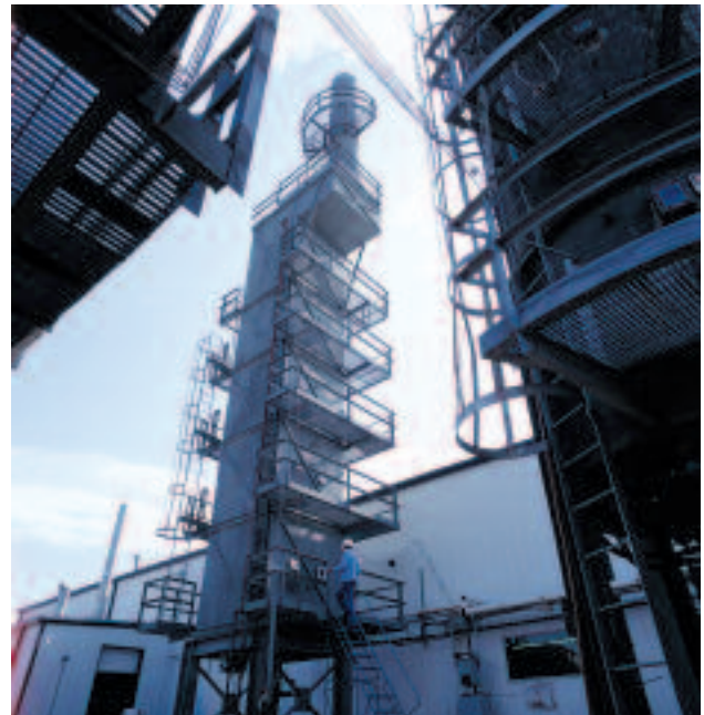
Burner research facility
