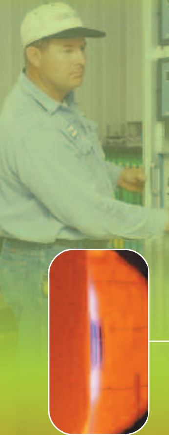
Radiant Wall Burner in Side-Fired Cracking Furnace
