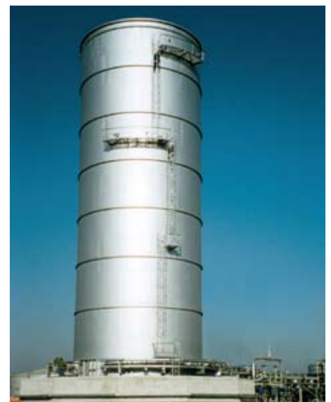
Totally Enclosed Ground Flare
