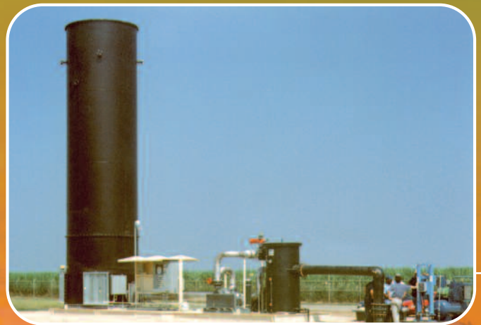
Biogas/Landfill Combustion System
